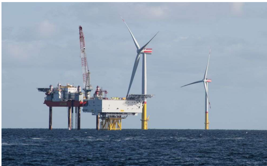
Wind farms are more expensive to build offshore than on land. But offshore wind farms can use larger turbines to generate more power. Pictured: Wind farm construction in the Baltic Sea
