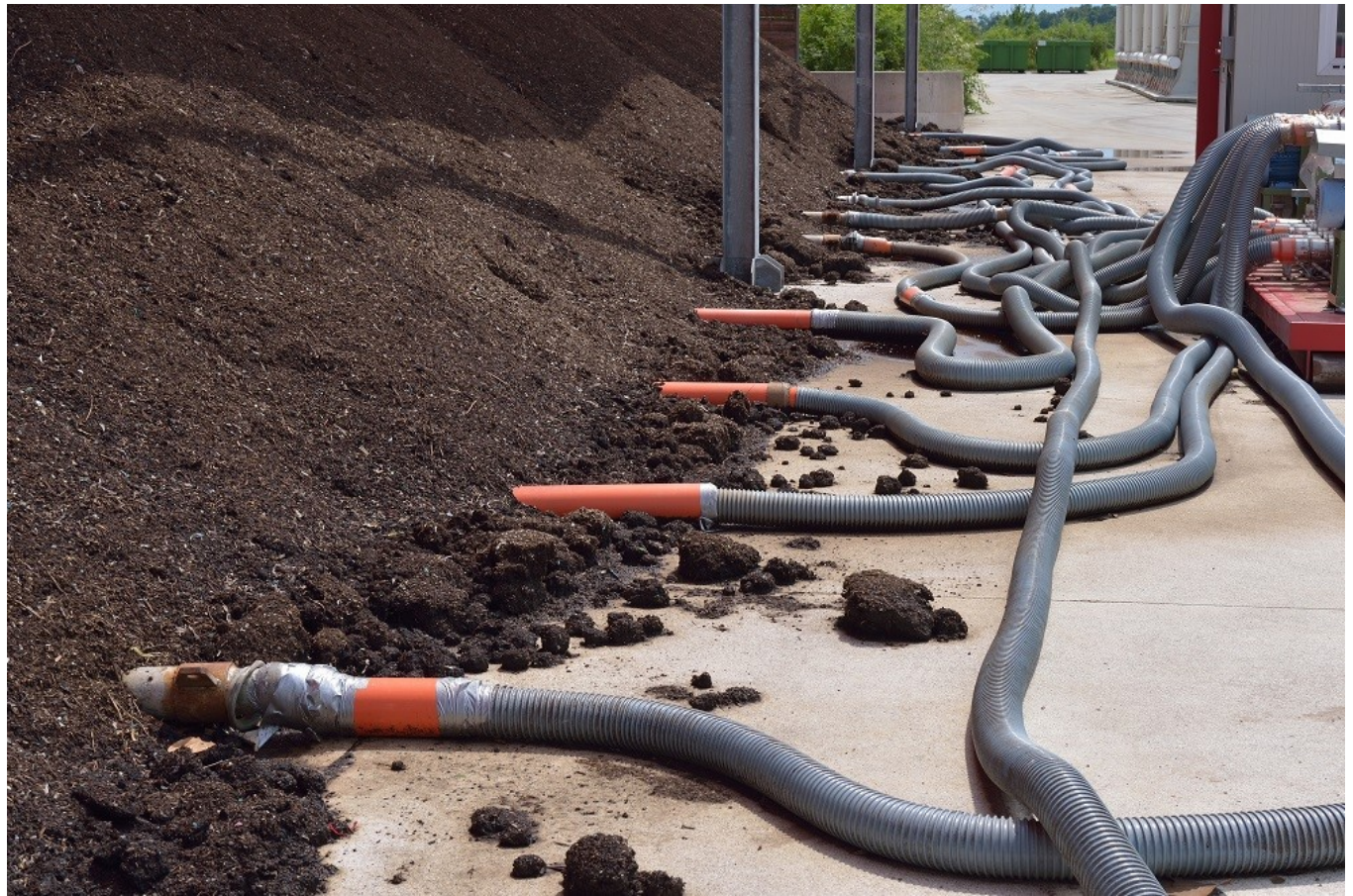
Industrial compost heap with aeration pipes. Image: Adobe Stock
