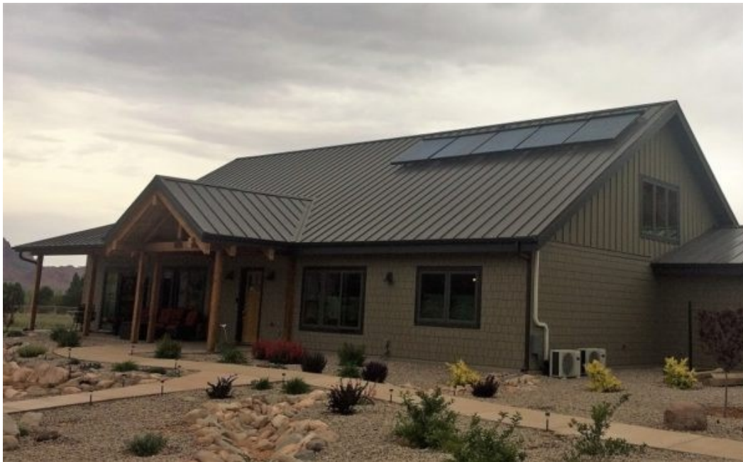
SOLAR WATER HEATING INSTALLATION AT CANYON NEST BED AND BREAKFAST IN MOAB, UTAH. IMAGE: SILK ROAD ENVIRONMENTAL
